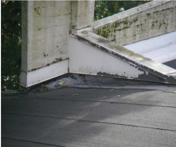
Triangular parapets on the roof at the East and West Elevations – South end.
