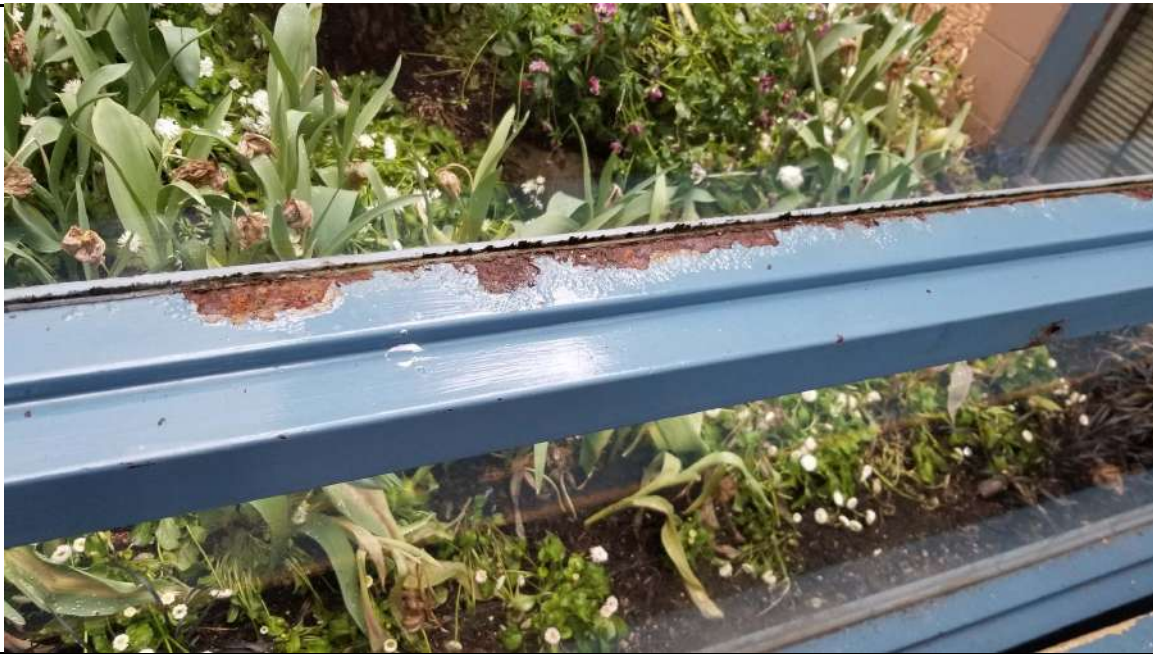
Photograph 1: Main Lobby and Concourse 101 - Flaking/Delaminating Lead Paint on Exterior Metal Window Frame
