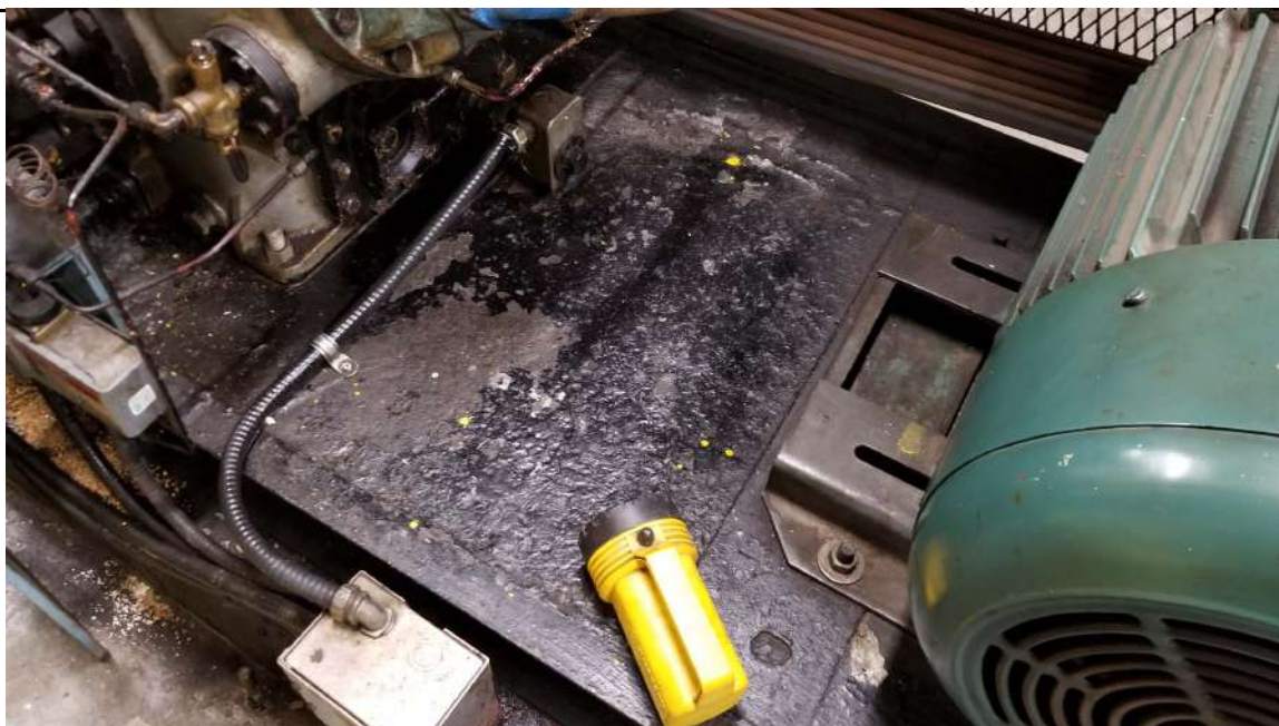
Photograph 5: Ice Plant (Engine Room) 126 - Flaking/Delaminating Lead Paint on Raised Concrete Bases at Centre of Room
