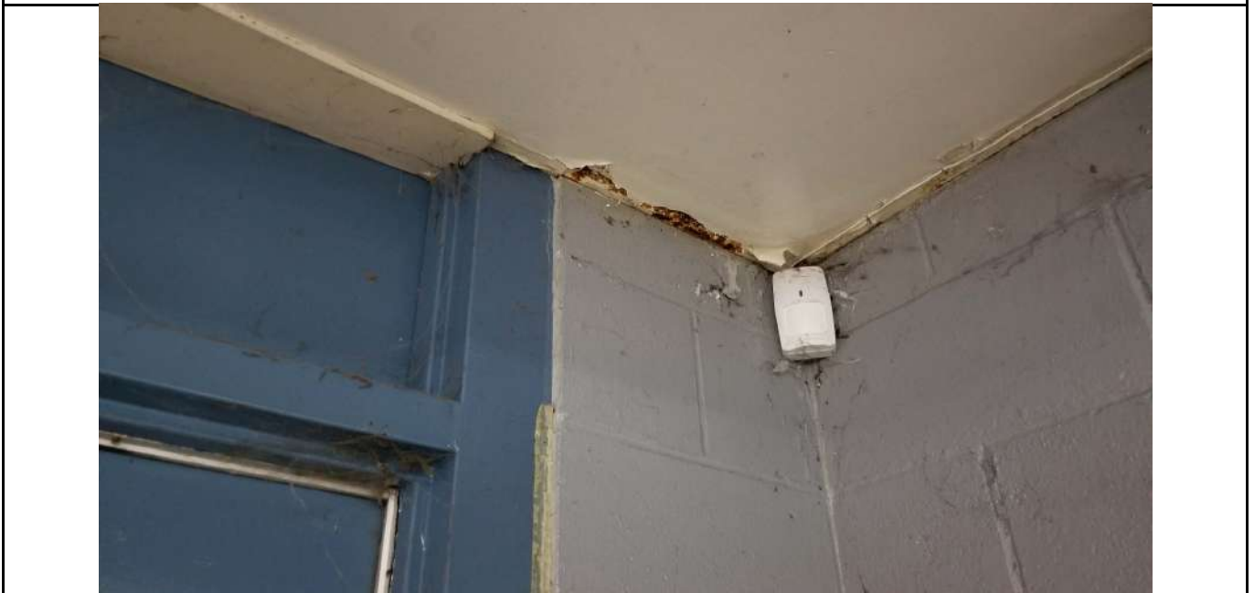
Photograph 8: Open Rink Area 121 - Damaged Asbestos Containing Filling Compound and Lead Paint on Gypsum Board Ceiling at Underside of Mezzanine Goal Crease Room 122, and Flaking/Delaminating Lead Paint on Concrete Block Wall
