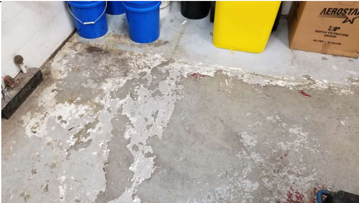
Photograph 2: Ice Plant (Engine Room) 126 - Flaking/Delaminating Lead Paint on Concrete Floor
