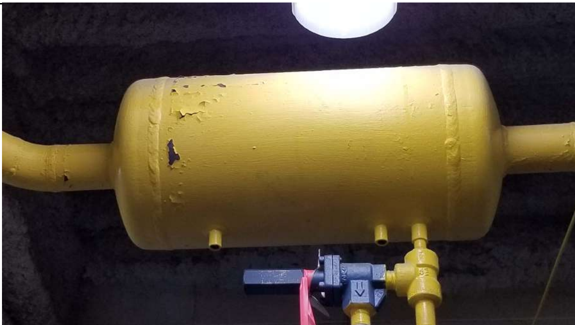
Photograph 4: Ice Plant (Engine Room) 126 - Flaking/Delaminating Lead Paint on Metal Piping above Pump at Centre of Room
