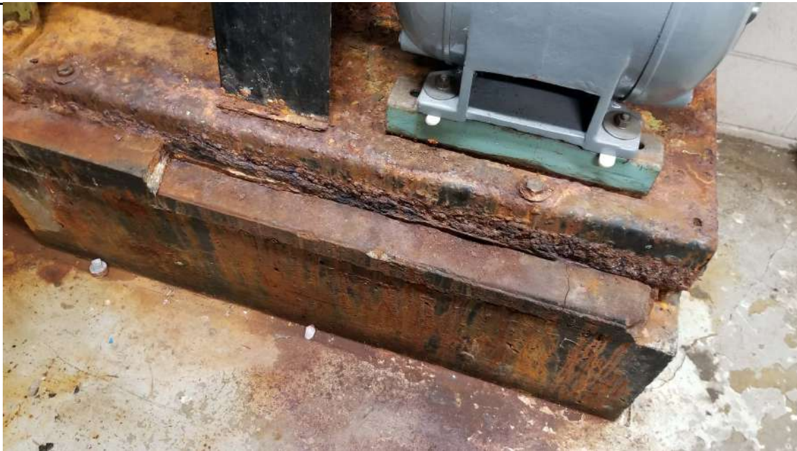
Photograph 3: Ice Plant (Engine Room) 126 - Flaking/Delaminating Lead Paint on Metal Base at Motor near West Wall
