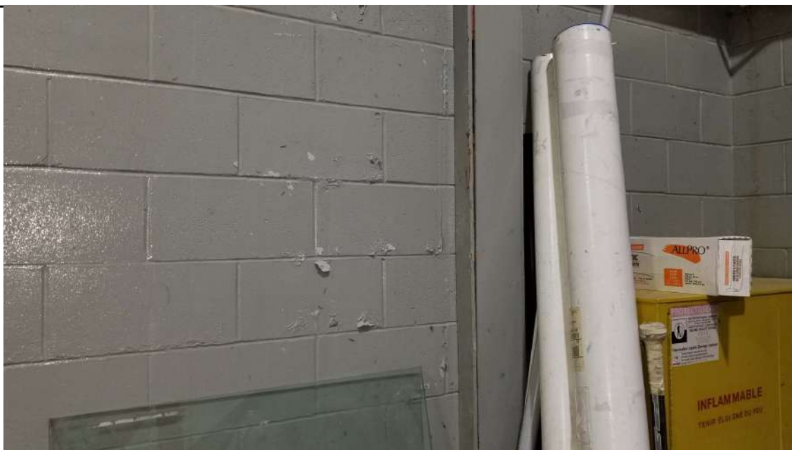
Photograph 6: Open Rink Area 121 - Flaking/Delaminating Lead Paint on Concrete Block Wall (near Northeast Corner)
