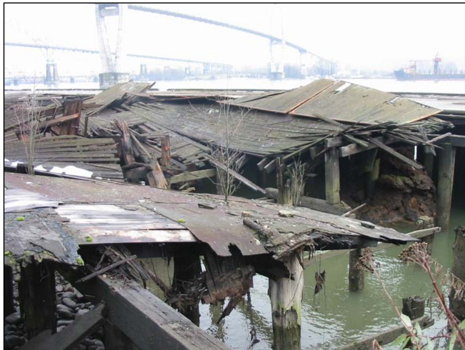
Photograph 4: The collapsed section of wharf toward the northwest of the Site
