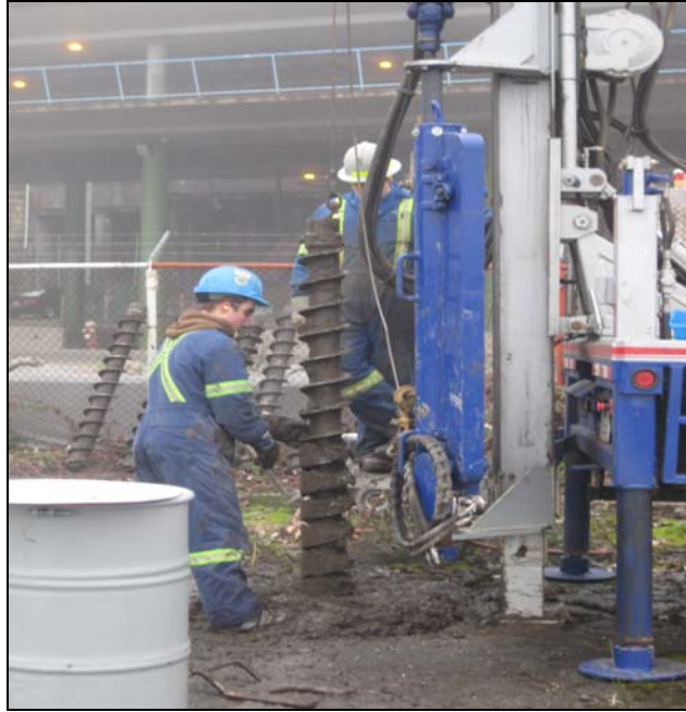
Photograph 5: Showing drilling in progress on the Site (hollow stem auger with a truck mounted drill rig)
